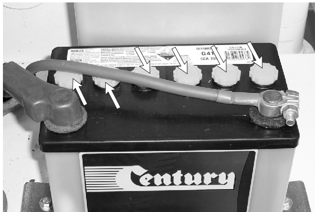
Figure 7.7 - Battery Fluid Level
