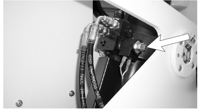
Figure 7.21.1 - Emergency Lower Valve, Controlling Lower Boom
