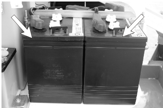
Figure 11.6 - Two DC Motor Batteries (Petrol/Diesel Engine Side)
