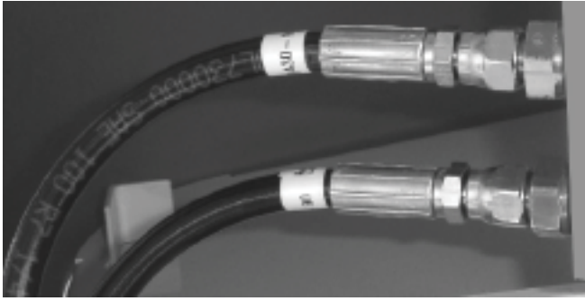
Figure 7.10 - Hydraulic Oil Leaks At Fittings And Hoses
