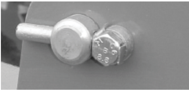
Figure 7.11 - Critical Pin Retainer Bolts
