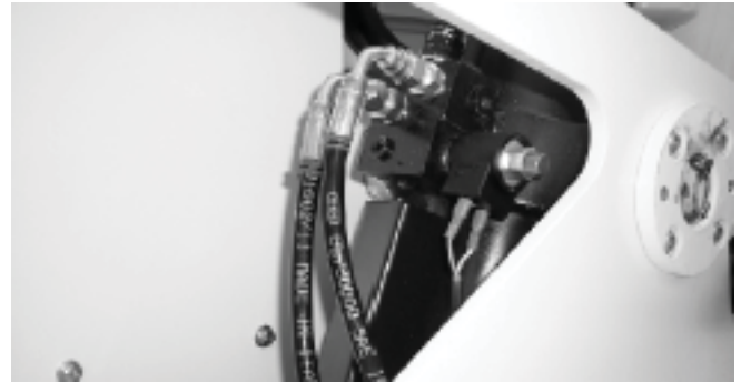
Figure 7.21.1 - Emergency Lower Valve, Controlling Lower Boom
