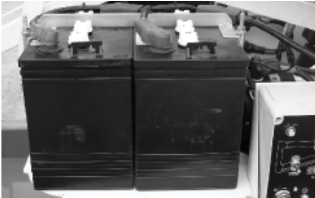
Figure 11.5 - Two DC Motor Batteries (Lower Control Box Side)
