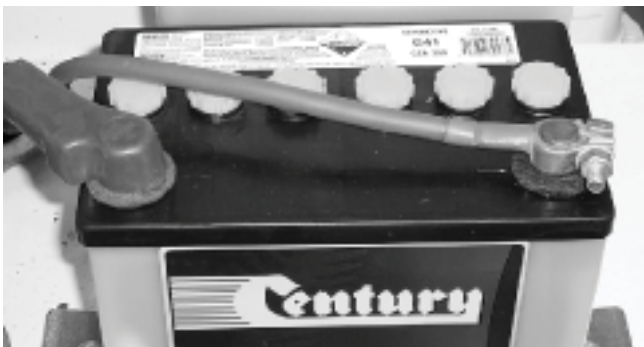
Figure 7.7 - Battery Fluid Level
