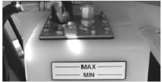
Figure 7.8 - Hydraulic Oil Level
